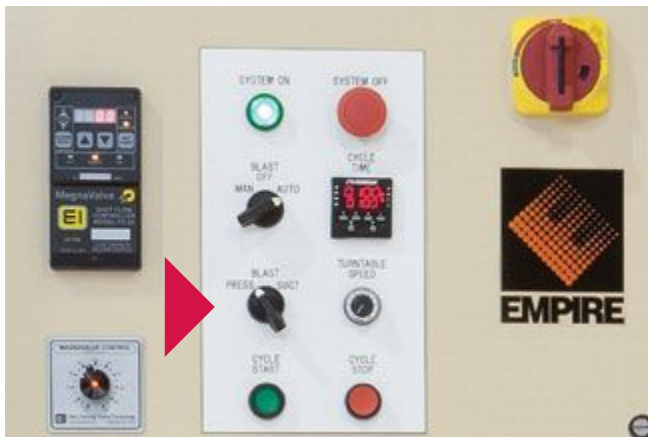
Figure 3. A selector dial for "PRESS" or "SUCT" on the system's control panel permits the operator to select pressure or suction blasting.
